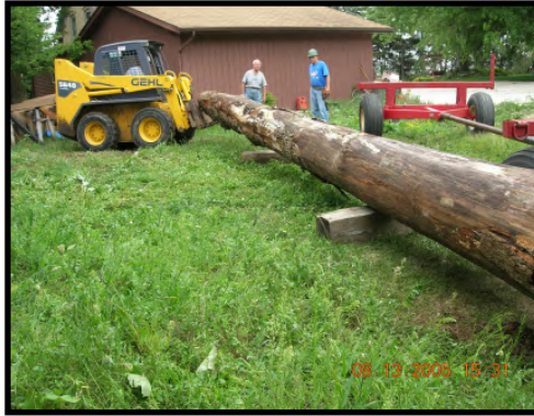
This is the red oak tree to be used as the base beam on the south side of the Lutze Housebarn. 2005
